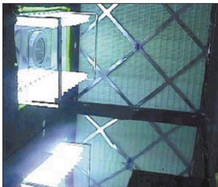
PHOTO A. UVGI array used for air disinfection. Note the specular reflective surfaces. Photo courtesy of Lumalier Inc., Memphis.
